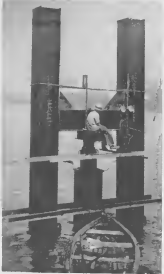
Not fishing but testing. The center pile is being jacked downward by this workman, but it is firm enough to raise the other reactionary piles instead.
